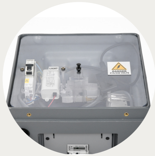
Internal Perspex insulating tray separating 240v from 12v hardware.
